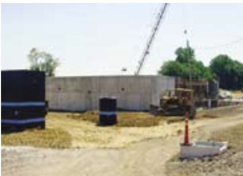
Sewer Treatment Plant
